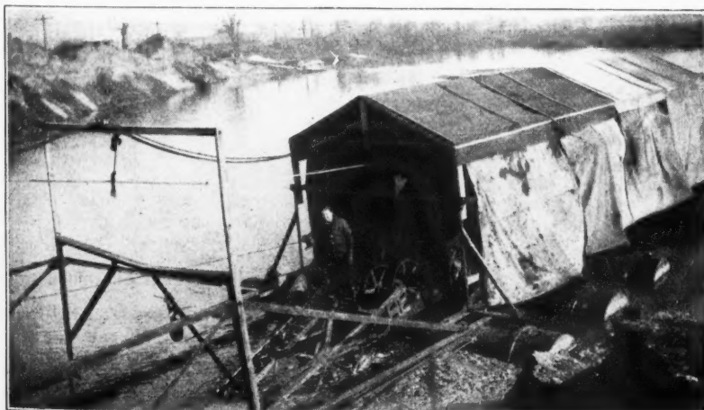
Close Up of Front End of Barge at Morristown. Note Barge Floating on Steel Tanks
